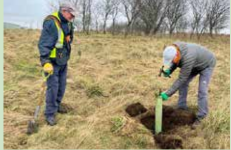
Team members involved in laying drainage channel and reinforcing the path surface
